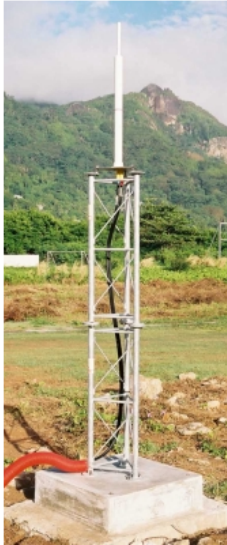
2m tower on concrete structure
